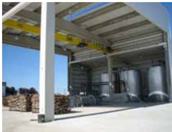
Fig. 1: ECOTRAFOR plant in San Vicente de Alcántara (Badajoz, Spain)
