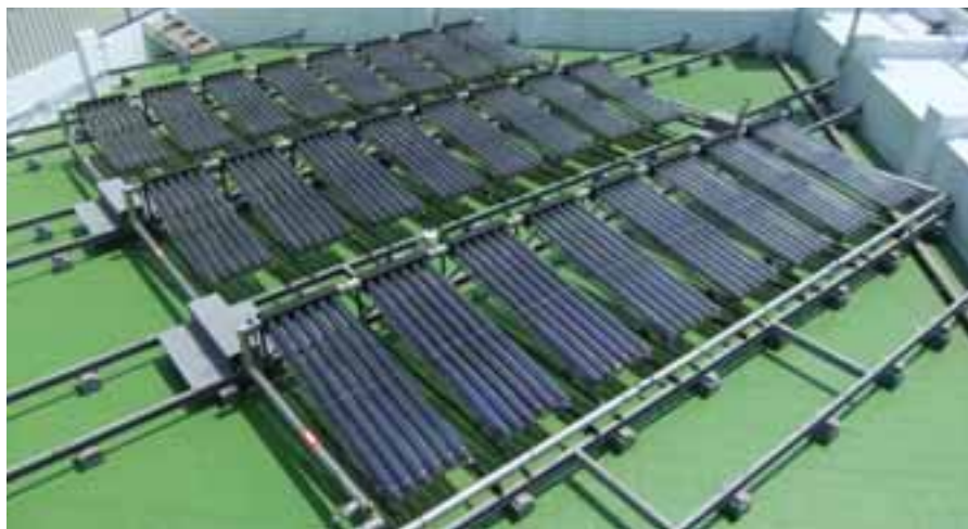
Fig. 1: Solar heating system used in present study
