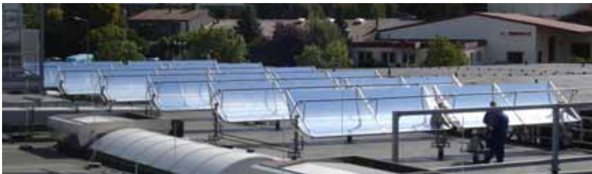
Fig. 1: Solar field with PTC1800 parabolic trough collectors
