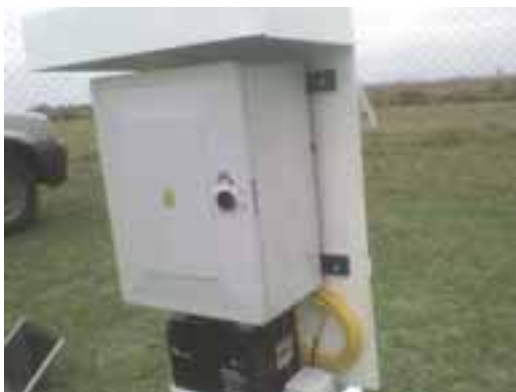
Fig. 2: Measuring station before placing exterior cover.
