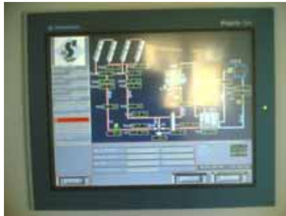
Fig. 4: SOLITEM Online Monitoring System at SOLTRIGEN
