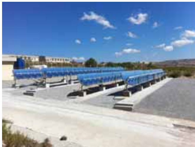
Fig. 1: The SOLTRIGEN Collector Field with SOLITEM PTC 1800 collectors
