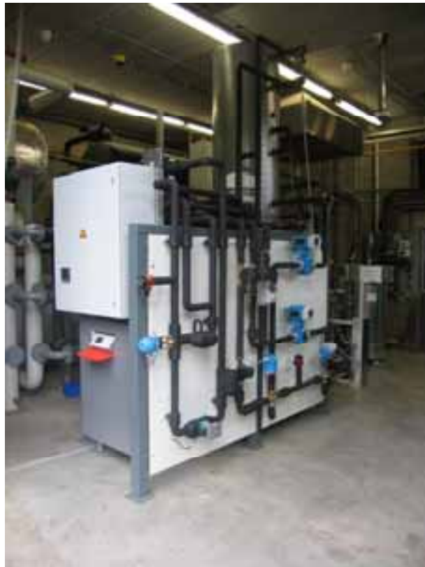
Figure 2: Picture of the heat pump installation
