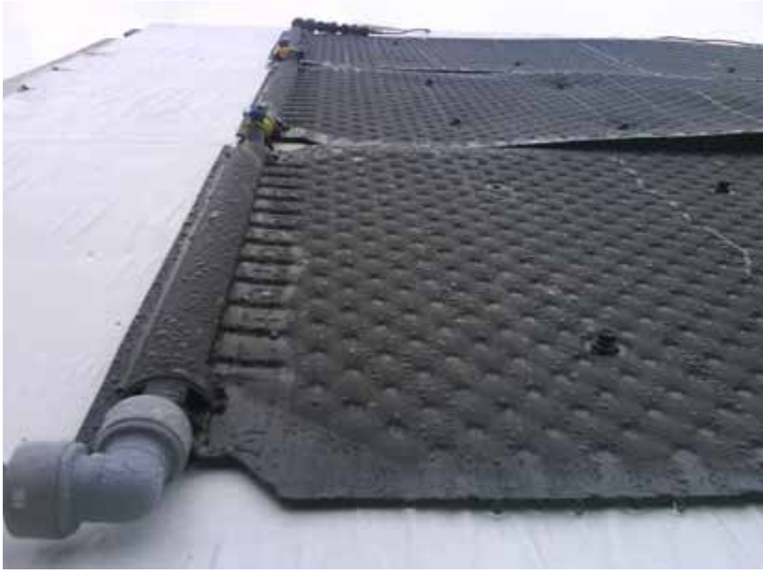
Fig. 3: Close up of the absorber showing the connecting pipe and header along the left side of the collector. The mounting screws to the roof can also be seen. It is assumed while modeling that no large amount of air flow can go behind the collector, so that a one sided operation/condensation can be expected. In a real situation a “two sided” mounting arrangement allowing air behind the collector may increase the performance during low temperature operation. (Photo from SP)
