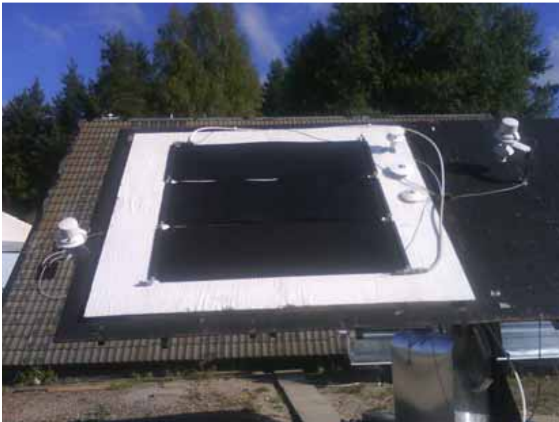
Fig. 1: The unglazed solar collector on the test stand with extra sensors for humidity, wind speed and air temperature. Also sensors for solar radiation and long-wave thermal sky radiation in the collector plane can be seen to the right of the collector. In the upper right corner a new kind of wind sensor is located. (Photo from SP)
