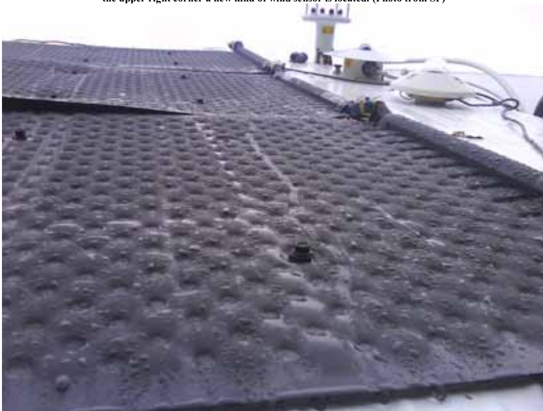
Fig. 2: Close up of the collector absorber surface during condensation operation. A lot of water is “produced” so it is important to have a really water tight roof under the collector. Here the inactive round welding spots on the absorber can be seen too. This affects the parameter values somewhat from the ideal numbers. (Photo from SP)
