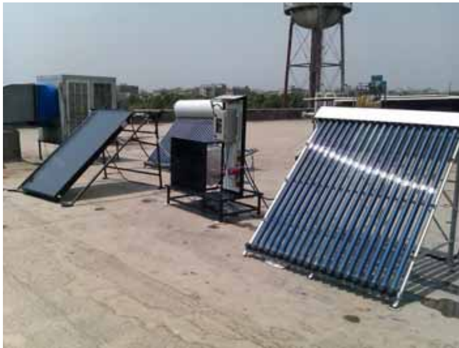
Fig. 5: collector and test facilities used for testing system and collectors
