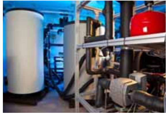
Fig. 7: Store test integrated into the system test facility
