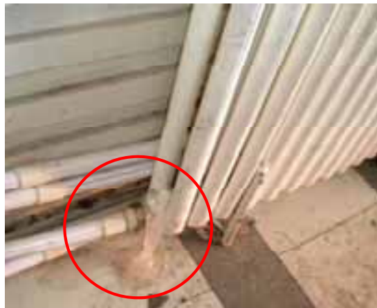
Fig.4: Frozen crack on the radiator
