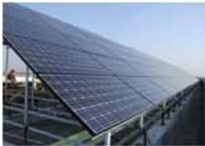
(a) Photo of the installed PV system
