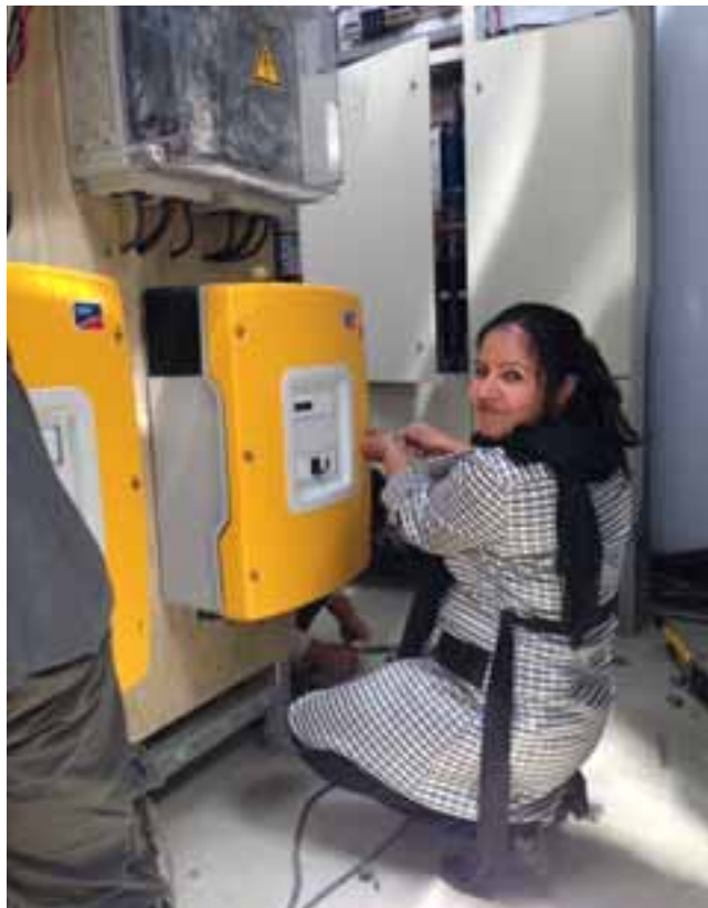
Fig. 6: SESI trained and utilized Afghan women technicians as part of the installation crew.
