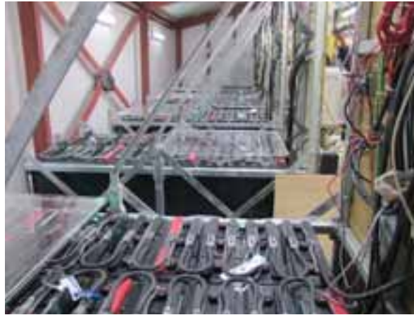
Fig. 3: Crown Battery Banks each at 48 V; 3,747 Ah at a C/20 Discharge Rate
