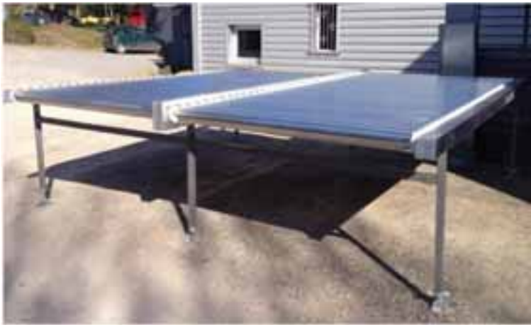
Fig. 8: Pilot ground mounted installation
