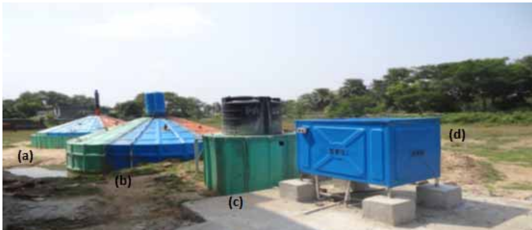
Fig. 2: Components of the AD system: gas chamber (a), main digester (b), predigester (c), chopper/grinder (d).
