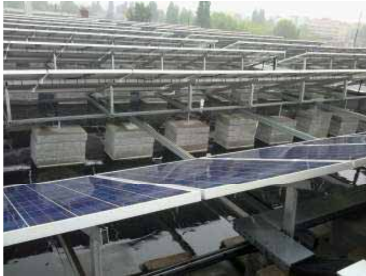
Fig. 2: The examined reference power plant
