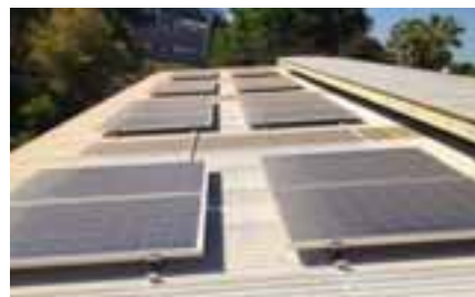
Fig. 2: The installed 5.0 kWp c-Si rooftop system (Auxin AXN-P6T275, Inverter: SunnyBoy SMA SB 5000TL-20)
