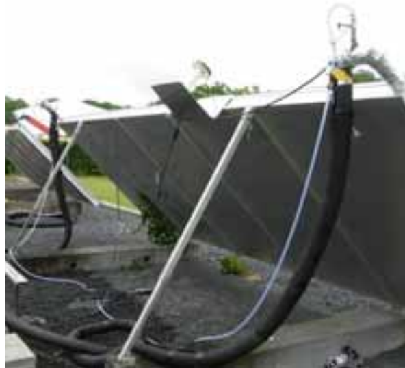
Figure 2: Solar collector HT-SA 35/10 used for the validation and plastic pipes arrangement for pressure drop measurement.
