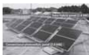
Fig. 3: Appearance of solar hybrid system
