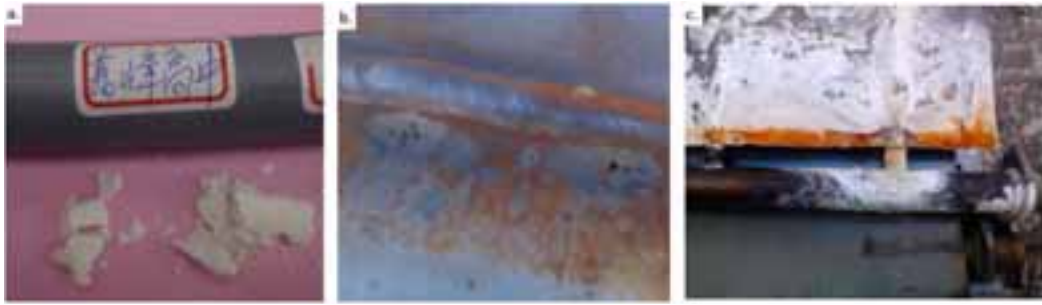
Fig. 2: (a) scaling of the connecting pipe; (b) pitting near the weld on storage tank; and (c) corrosion and scaling on solar collector plate.
