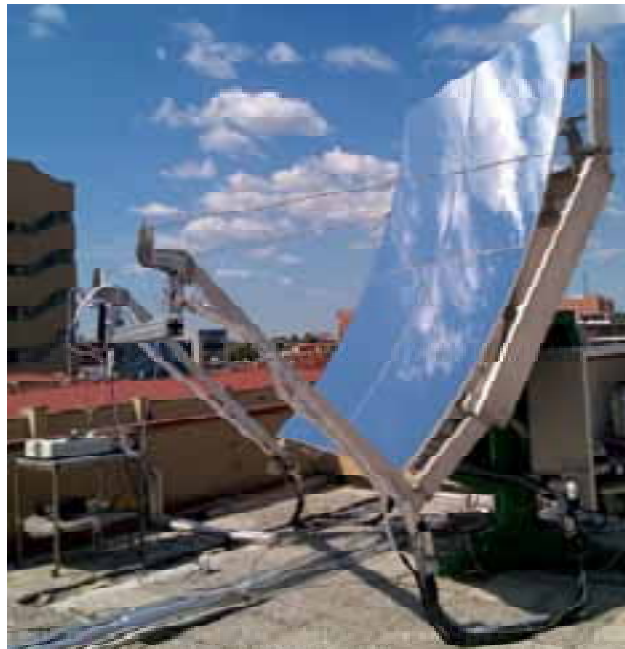
Fig. 1: Prototype of the asymmetrical parabolic trough linear solar concentrator and solar flux map measuring system installed at the Solar Energy Conversion Lab of the University of Padova.
