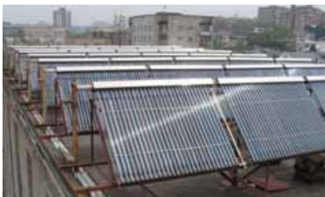
Fig. 1 - General view of the experimental SWHS, its solar collectors (roof of the Far Eastern Federal University, campus building)
