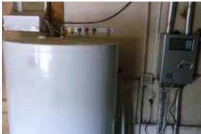
Fig. 2: The tank and controller of system
