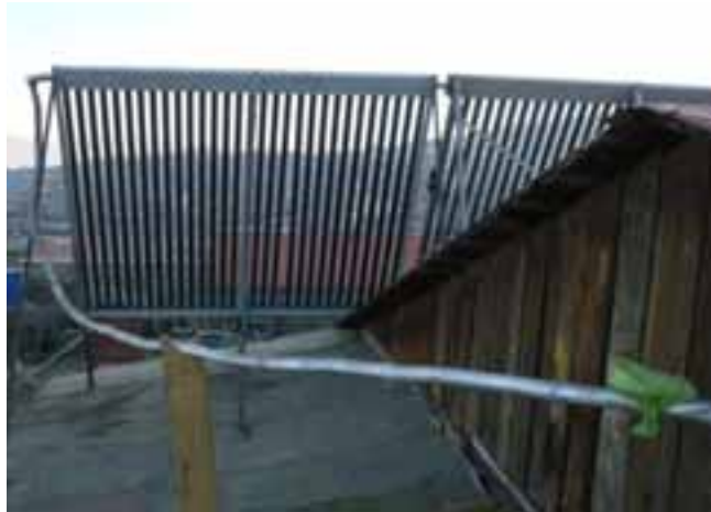
Fig. 3: Solar circuit pipe to return
