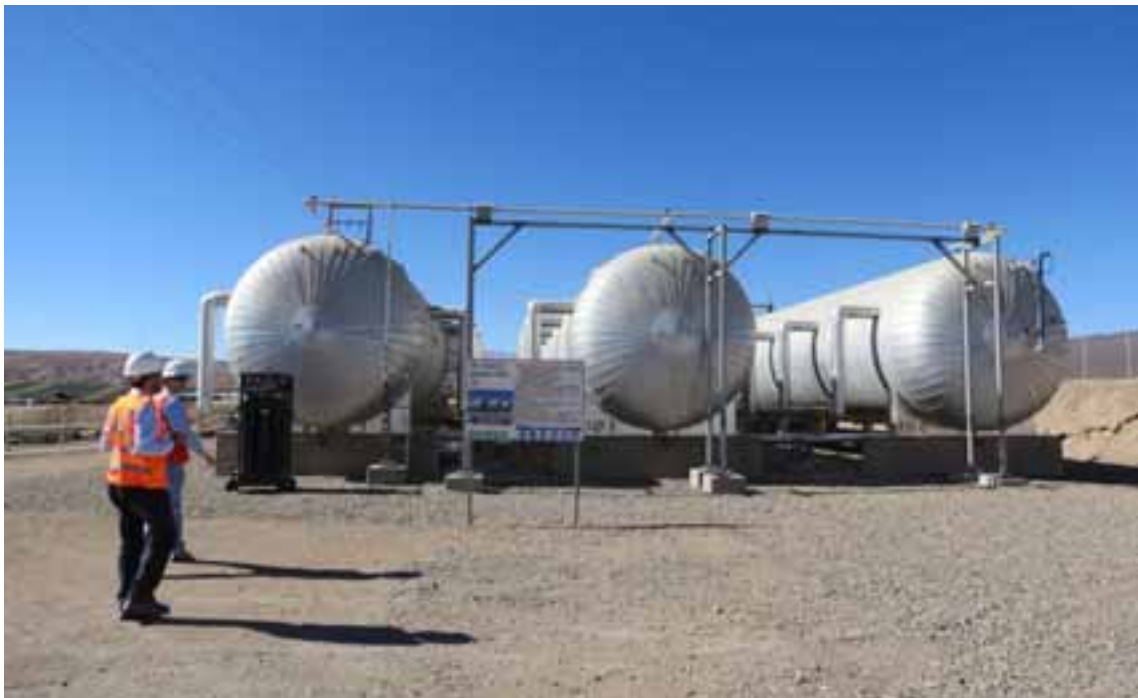
Fig. 6 The “Centinela” parabolic system storage tanks. Each has a capacity of 120 m 3
