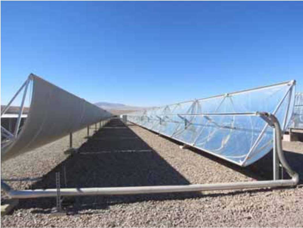
Fig. 5 The “Centinela” parabolic trough plant. The tracking is east-west
