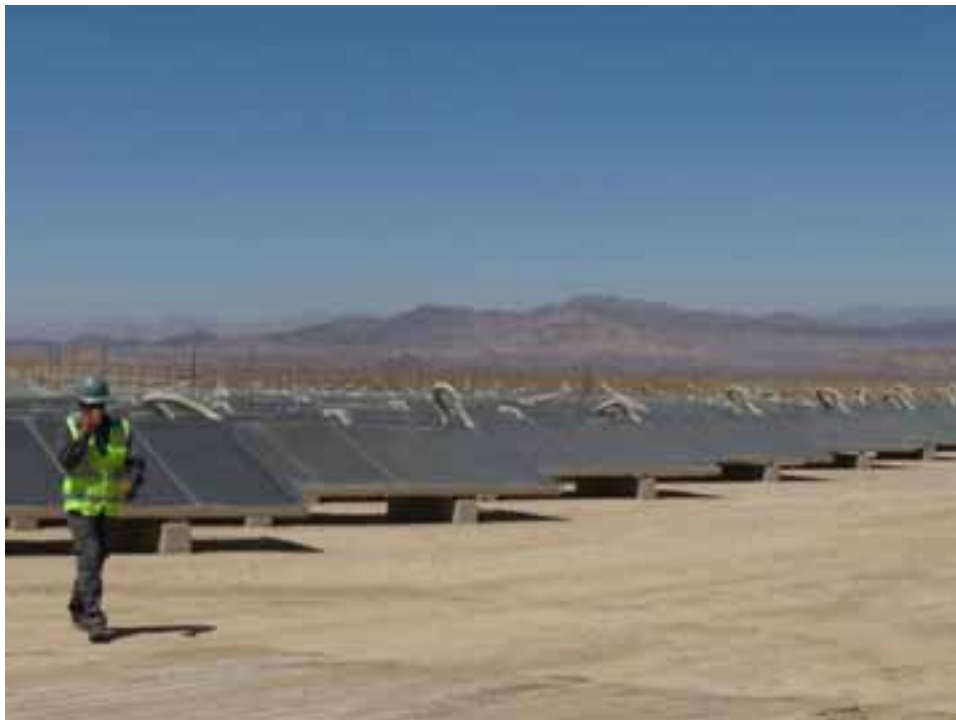
Fig. 5 Part of the flat plate collector field at “Pampa Elvira”. The tilt mechanisms can be seen
