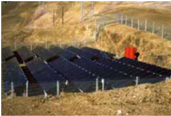
Fig. 2 The flat plate collector field in El Salvador (1982)
