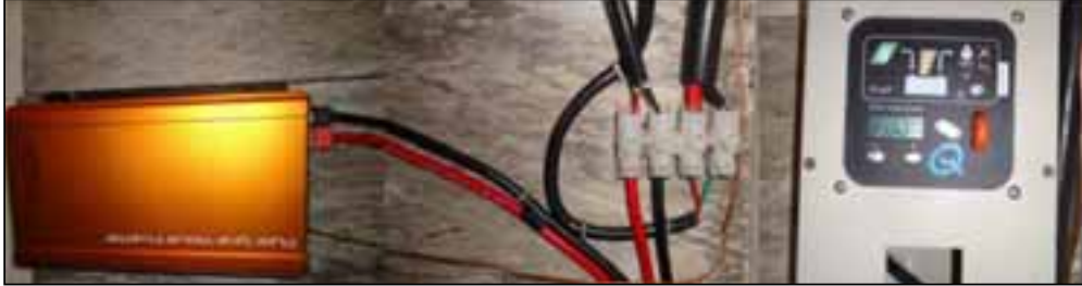
Figure 3: Typical installation of prepaid system and inverter.
