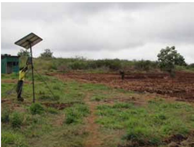
Fig. 9: Thika solar water pumping system used for drip irrigation.
