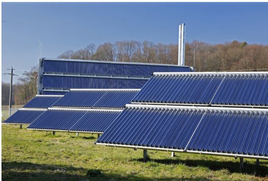
Figure 3: Vacuum tube collectors in Büsingen, Germany
