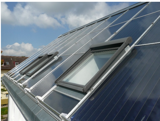
Figure 5: Roof integrated solar thermal collectors on "solar@home"-building in Crailsheim, Germany
