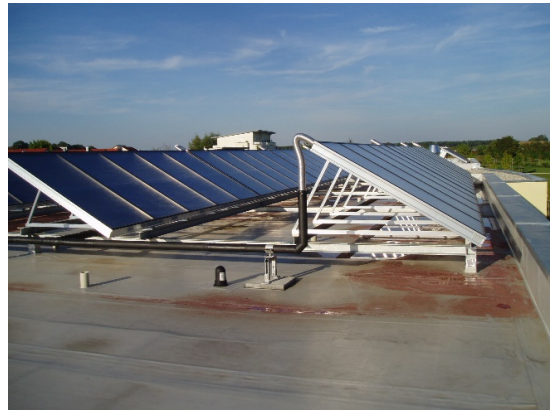
Figure 6: Solar collectors elevated on flat roof in Neckarsulm, Germany
