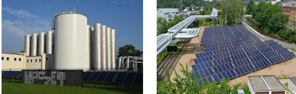
Fig. 3: South solar collector field and two-zone storage (left) and north collector field (right) in the Brühl system, Chemnitz.
