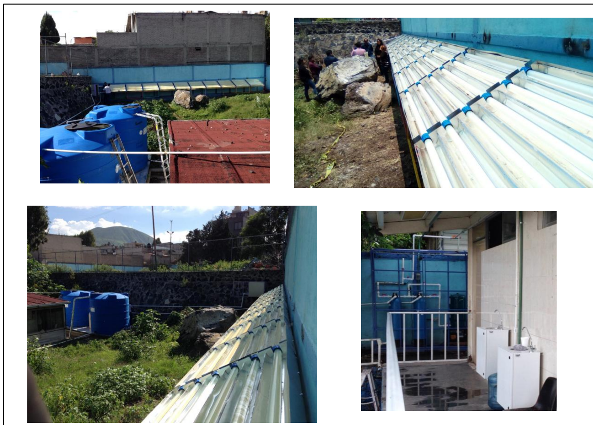
Fig. 14: Photochemical treatment system coupled to potable water train system and drinking water dispensers
