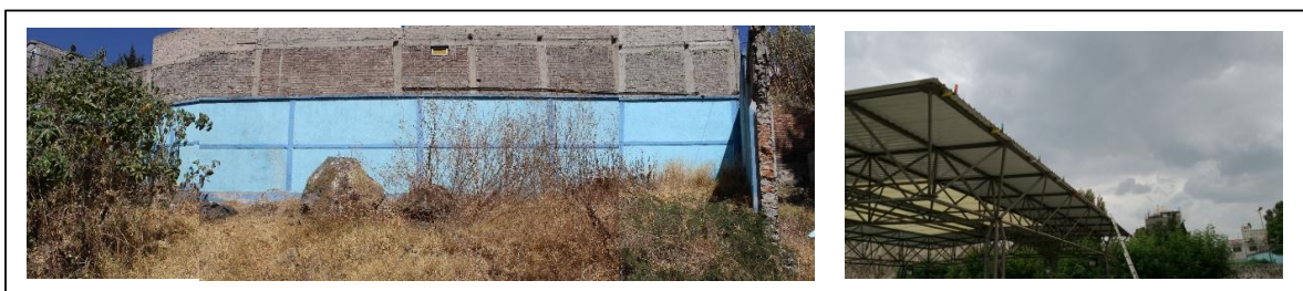
Fig. 5: Enclosing wall south oriented inside the school (left) and rainfall roof caption surface (right).
