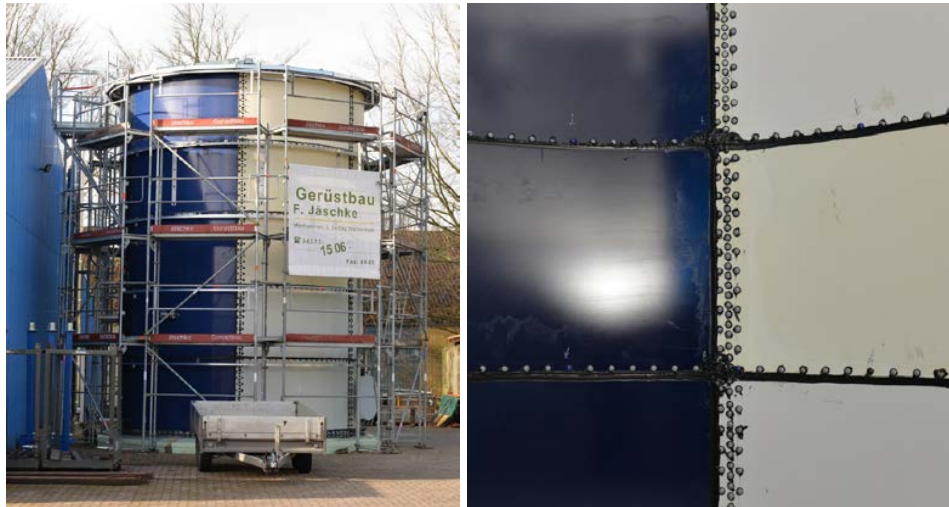
Figure 6: Demonstrator in Nortorf, Germany (left), approx. 100 m 3 , single-zone storage tank, test of different coatings, interior view (right), April 2016
