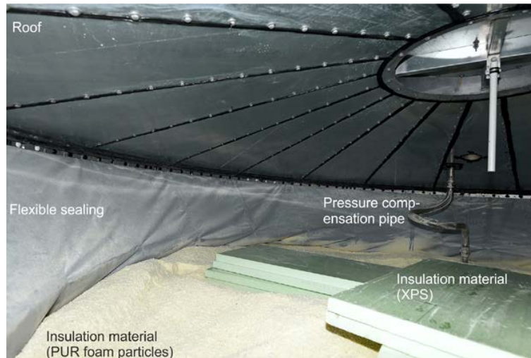
Figure 8: Laying of XPS panels on the PUR foam of the floating ceiling in the attic during the construction, July 2017
