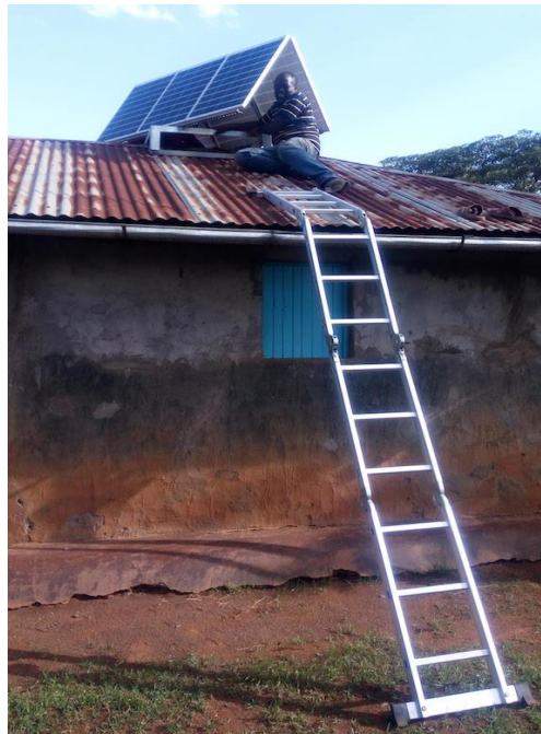
Figure 1. Rooftop PV Installation for Mogotio Dairy Farmer FMC
