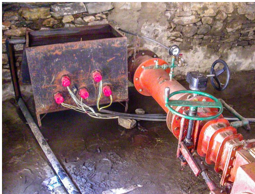
Fig. 2: Traditional water heater “dumb” dump load in MHP (micro-hydro-power) plant in Nepal
