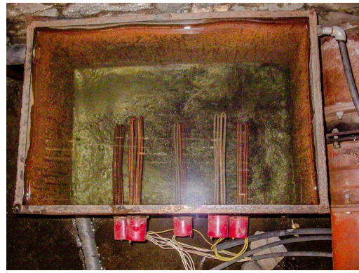
Fig. 3: Resistive water heater elements are used to dissipate energy into the turbine's exhaust water.
