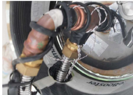
Fig. 16. Electrical tracer to the inlet and outlet pipe of the module.
