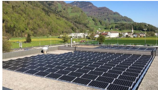
Figure 10: P&D project Lintharena in Näfels (CH). Uncovered PVT collectors for the pre-heating of groundwater providing heat to a heat pump (Rohrer, 2016).
