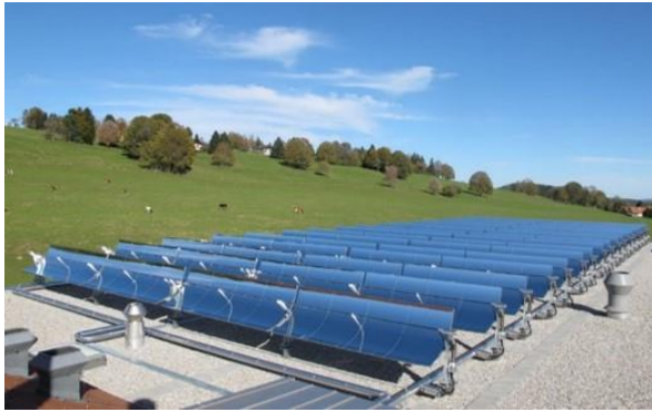
Fig. 1: SPHP in Saignelégier, 1000 m above sea level, 627 m 2 (aperture) PTC collectors with axis orientation NS with 18° deviation counterclockwise
