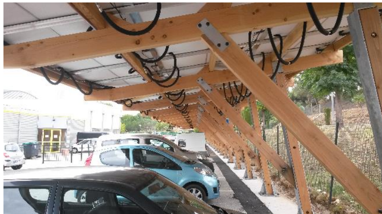
Fig. 3: picture of the PV/T canopy for the municipal swimming pool of Perpignan (France)
