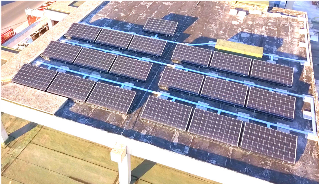
Fig. 3: Picture of 19 mono-crystalline photovoltaic modules (280 Watts peak (Wp) for each module) on the Atisys roof top
