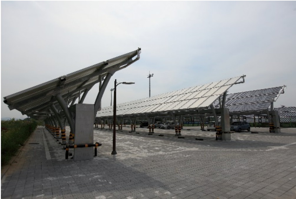
(a) Solar thermal collectors
