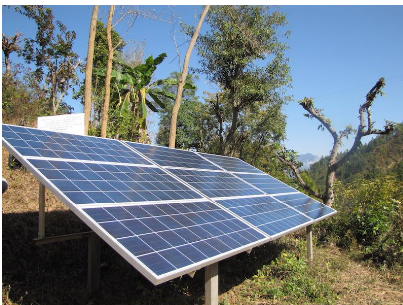
Fig. 7: Solar water pumping array (9s x 1p) rated at 1.26 kWp used for irrigation by the Taule village farmers.
