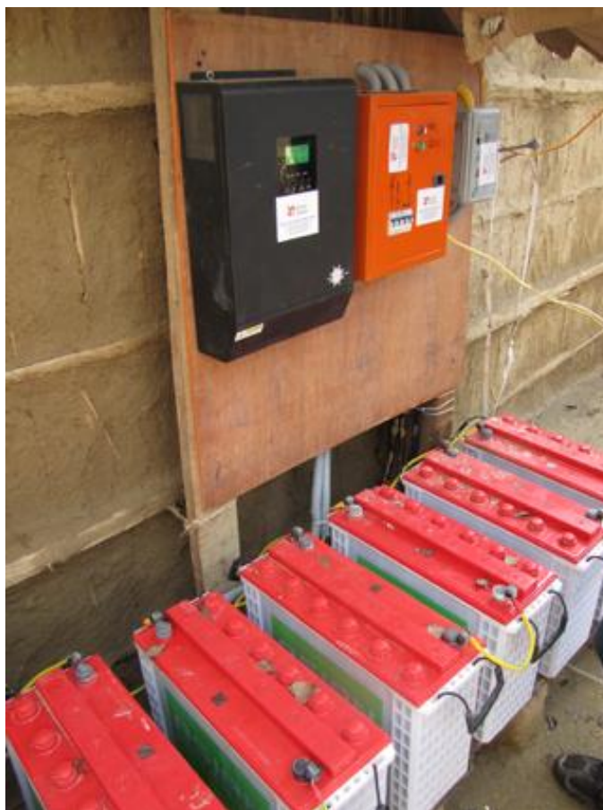
Fig. 13: Piparkoti village inverter and controls for large scale rice irrigation
