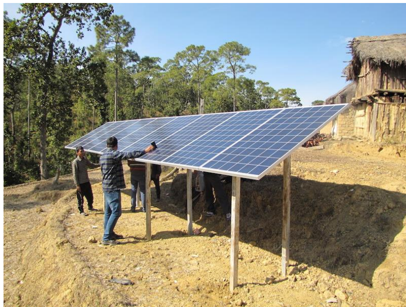
Figure 12: WI technicians measuring solar irradiance for the PVWP installed in Odaltal village of Surkhet District.
