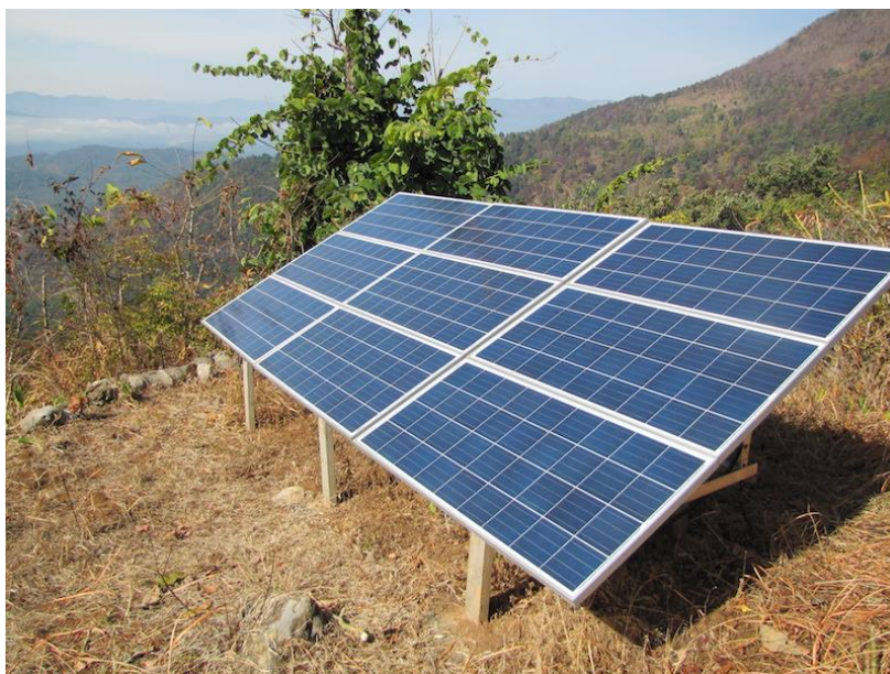
Figure 10: Solar power array using German made Komaes140 Wp PV modules (9s x 1p) for t Pokharikada using a Grundfos submersible centrifugal solar water pump.
