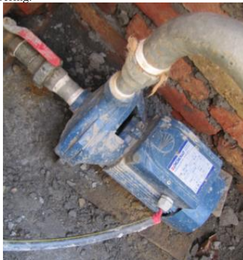
Fig. 2: Pedrollo (Italian) surface centrifugal AC solar pump used in Odaltal village of Surkhet District for rice irrigation.
