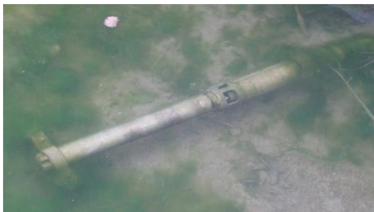
Fig. 3: Grundfos submersible centrifugal pump used in a river for Taule village.
