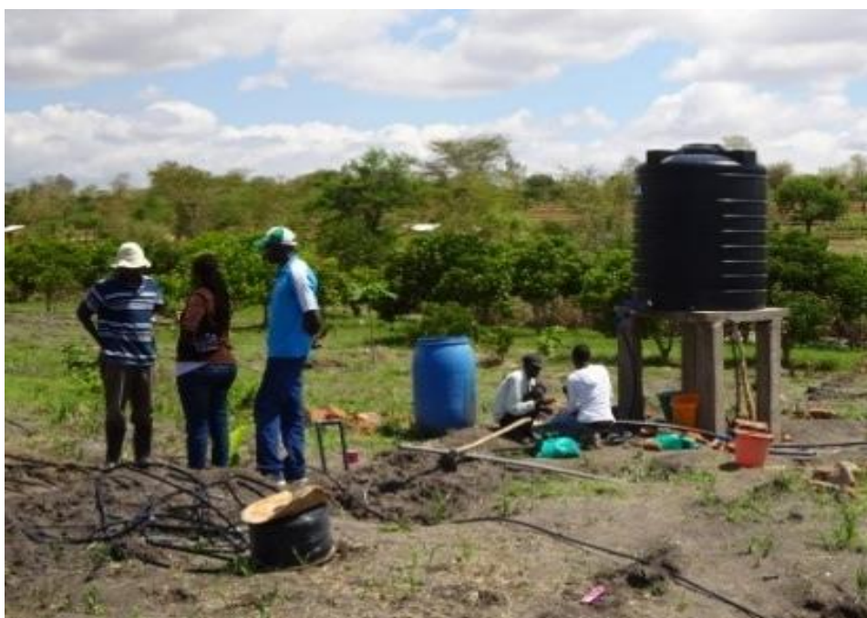
Fig. 7: Installation of water tank and drip lines at Shadrack Nzioka's farm.
