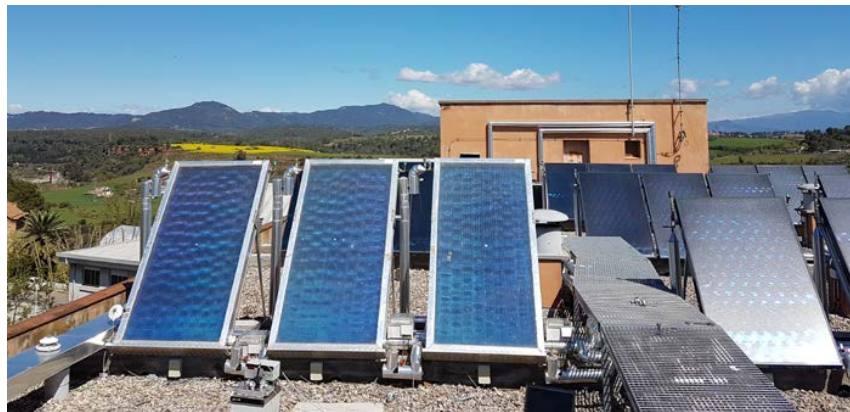
Fig. 12 Solar energy capturing field of the Albada Building in Parc Tauli Hospital. The three prototypes are tested alongside the conventional flat plate solar collectors without TIM.
