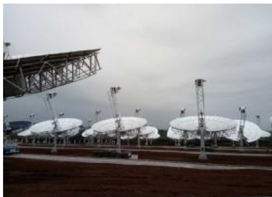
Fig. 10: Dish Stryn solar thermal power system in Tongchuan
