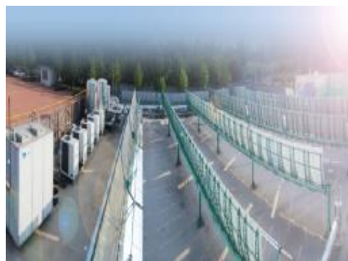
Fig.6: Parabolic-trough collectors for solar cooling
