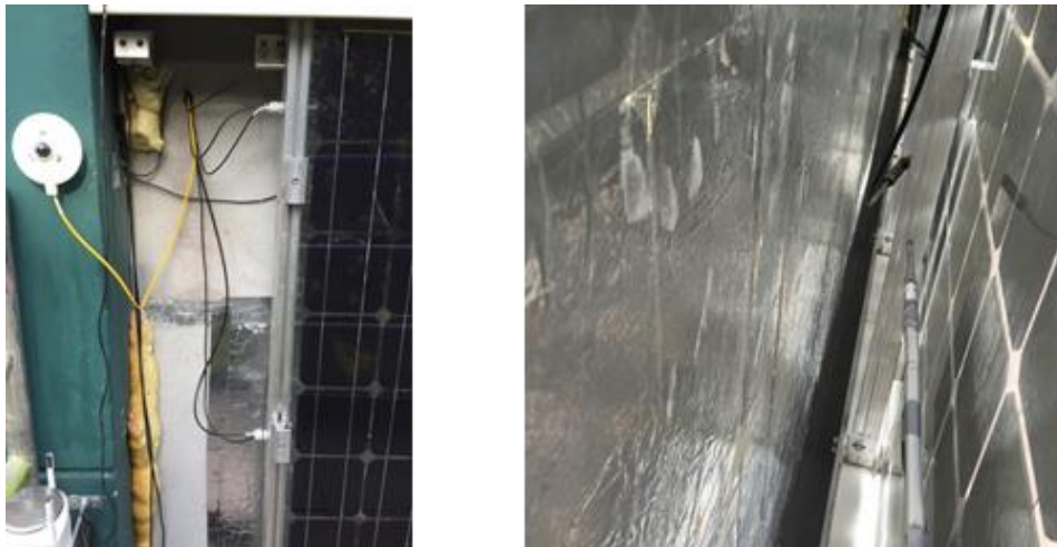
Fig. 6 Pyranometer and outdoor temperature sensor (left), anemometer and inner temperature sensors (right).
