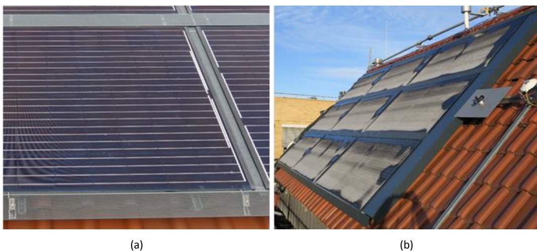
Figure 4: Perforated plates used to cover the gap between the single collectors of the PV-T field (a) and overall view of the PV-T field configuration with perforated and side plates (b)
