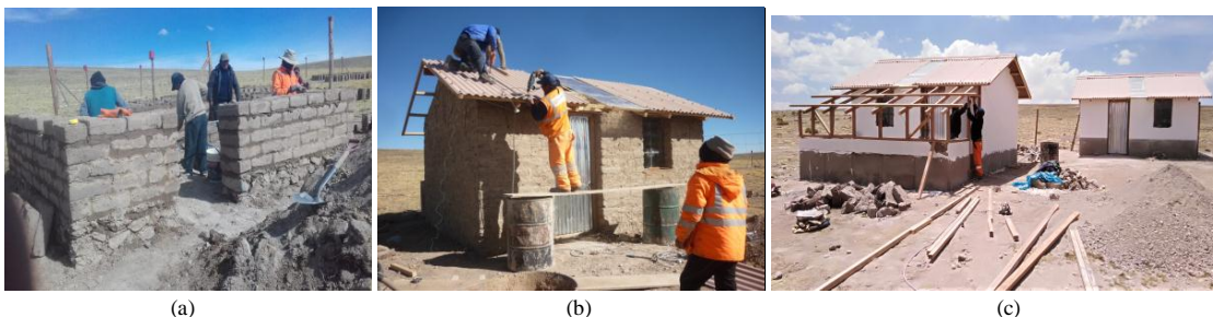
Fig. 2: Views of part of the construction process of the experimental modules, (a) adobe walls, (b) fiber cement roofs, and (c) wooden structure of the attached greenhouse (at ME2).
