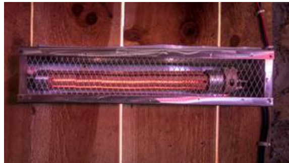
Fig. 12: Air Heater Resistor in the Community Center
