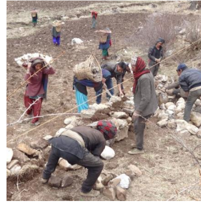
Fig. 14: Building Elevated Penstock
