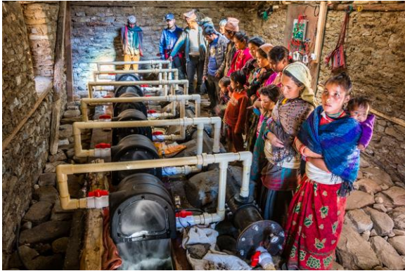
Fig 5: Six Turbines, Saddles, and CPVC Supply Lines
