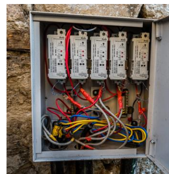
Fig 9: Junction Box with 3-Phase Buss Bar and Prepayment Meters
