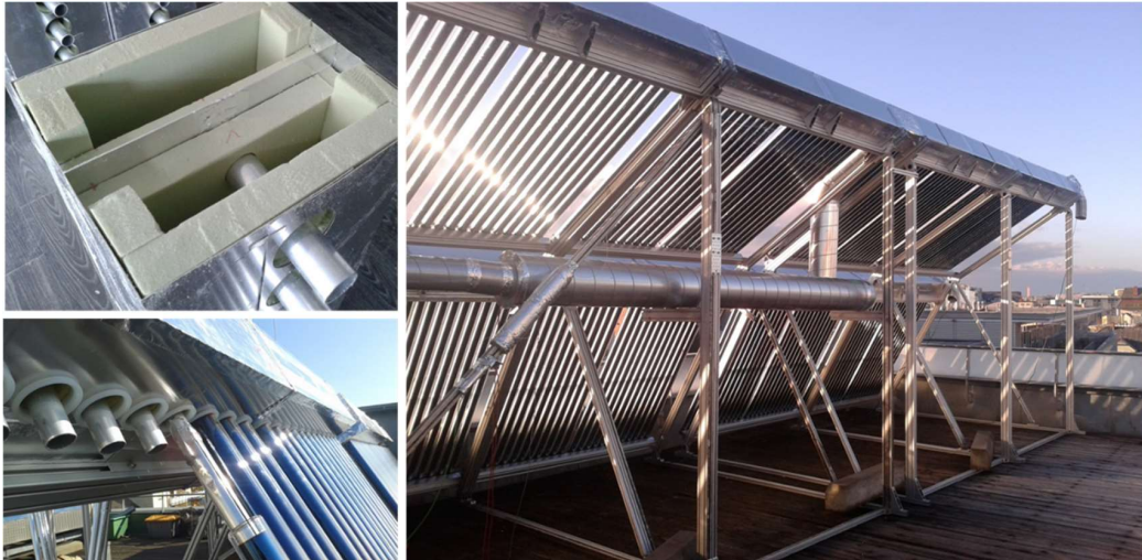
Fig. 7: Pictures of the installed solar hot air installation
