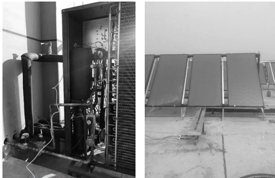
Fig. 5: Experimental dual source heat pump unit and solar collectors
