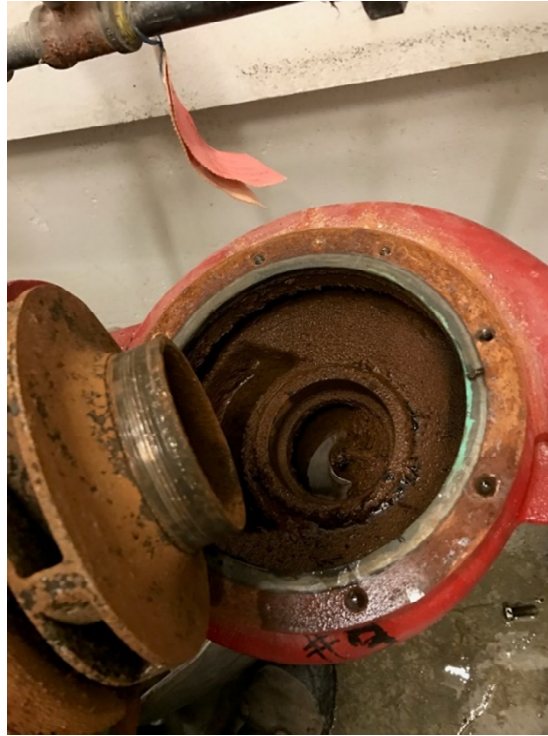
Fig.6: Pump impeller volute with corrosion deposits.
