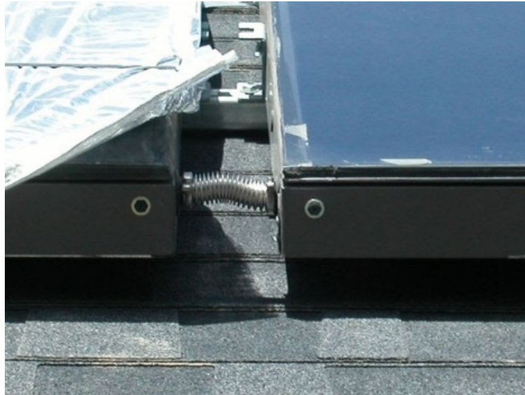
Fig. 5: Bowed bellow device between collectors.
