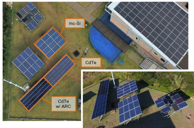
Fig. 1: Aerial view of the three PV systems located at the Fotovoltaica-UFSC research laboratory in Florianópolis, Brazil (27°S, 48°W) and used in the present study (mc-Si, CdTe and CdTe with ARC)
