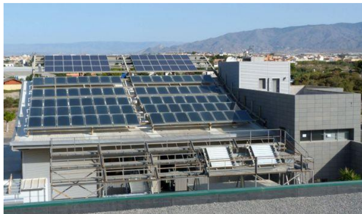
Fig. 1. Upper view of the photovoltaic system located on the roof of CIESOL building, at University of Almeria, Spain.
